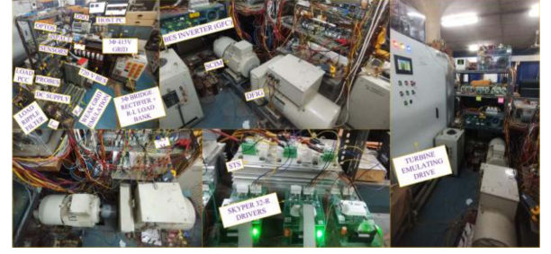
Fig. 10 Hardware setup of distributed wind microgrid with battery.
