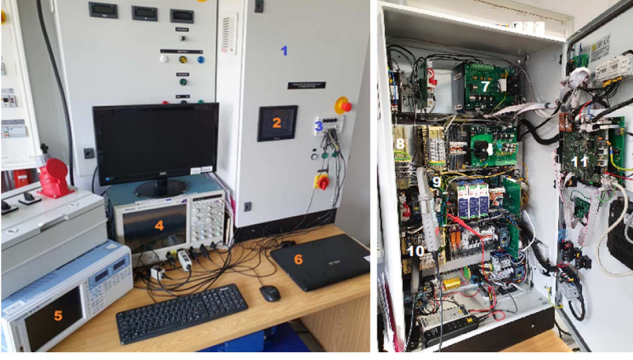
Fig. 31. Laboratory setup view: (1) converter cabinet, (2) HMI, (3) signal panel, (4) oscilloscope, (5) power analyzer, (6) programming laptop, (7) AC-DC converter, (8) LCL filter inductance L_2 , (9) LCL filter capacitance C , (10) LCL filter inductance L_1 , (11) main control board with DSP and FPGA.
