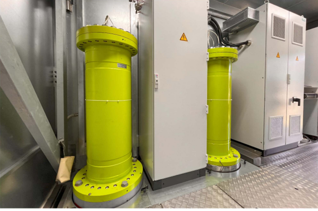
Fig. 4. Photograph of the Stormetic FESS with the two 60-kW flywheels.
