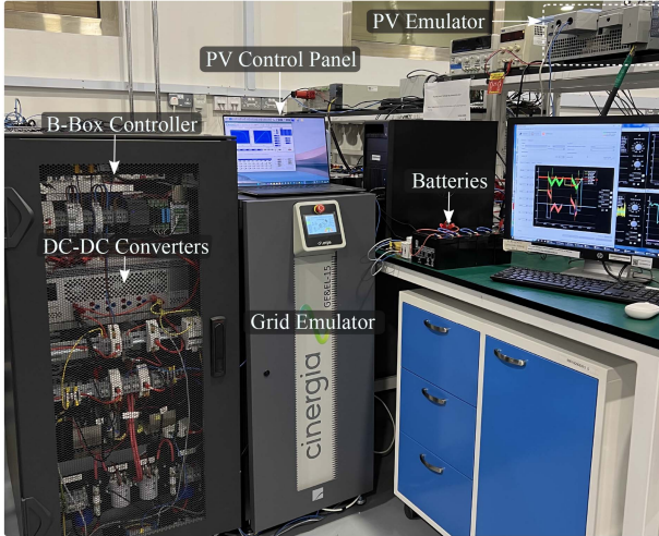
Fig. 6. Experimental hardware setup of the PV system with ESS.
