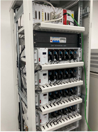
Fig. 15. Experimental MMC setup with an RTU-BOX204 controller (the top enclosure).
