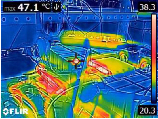
Fig. 31. Thermal testing results for the planar coupled inductor under 50 kW step-up case (900 V to 1 kV).
