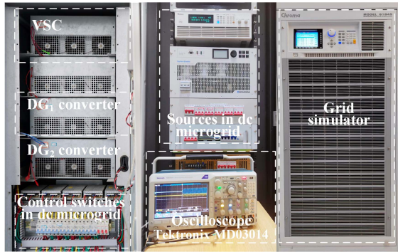
Fig. 38. Experimental setup of dc microgrid.
