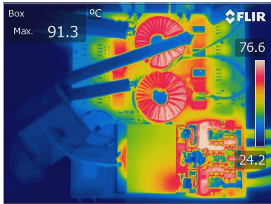
Fig. 27. Thermal test under rated input voltage and full load condition.
