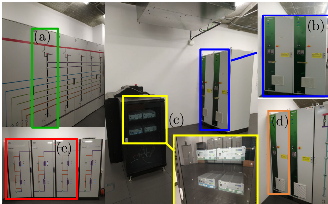
Fig. 27. Photographs of the laboratory. (a) AC busbars. (b) 15-kVA converters. (c) Real-time computers. (d) 75-kVA converter. (e) Line impedances.
