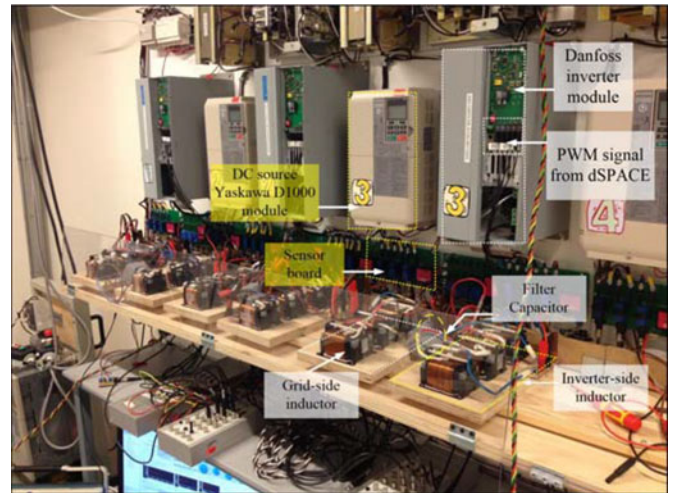
Fig. 27. Experiment setup photo with the three-phase grid inverter.
