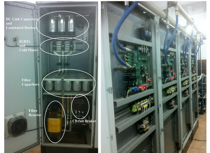
Fig. 17 Developed HAPF system, front view of a typical HAPF unit on the left, and rear view showing control PCBs and cooling water piping on the right.
