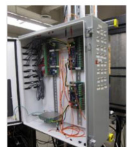
Fig. 18. (a) Simulator lab at Florida State University Center for Advanced Power Systems. (b) DAC card at the back of the RTDS rack. (c) DSP IoCU board analog inputs and outputs.
