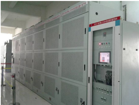
Fig. 20. Cascade STATCOM used to test the proposed control.
